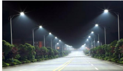
50,000 street lights and 6000 sign lights
